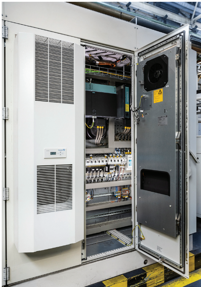
Picture above: Opened control cabinet with two X-Series cooling units DTI 6X1E.
