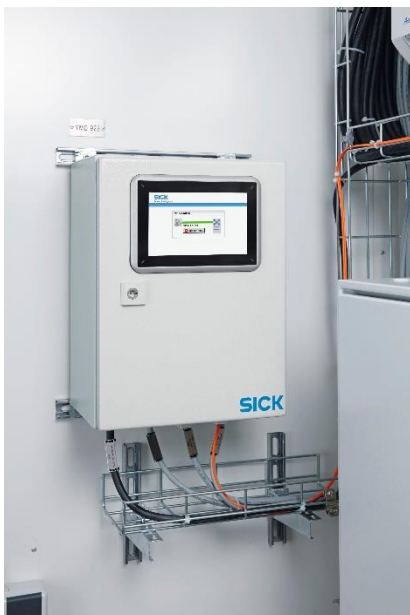
Photo caption: The Meeting Point Router (MPR) from SICK allows the communication-enabled cooling devices from Pfannenber to be serviced remotely from any location. Image © SICK AG.
