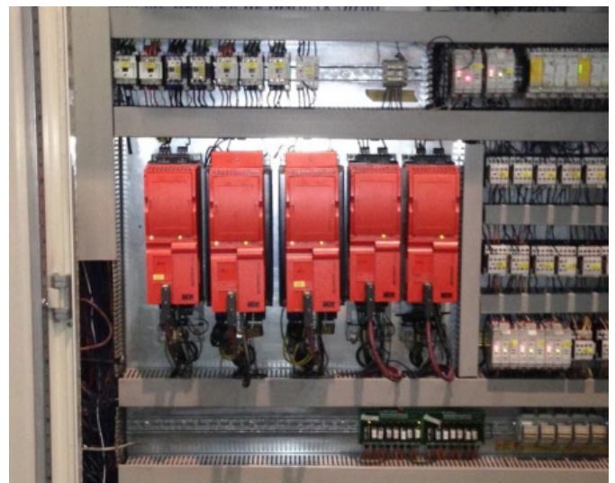
Very dirty frequency converters before cleaning (above). The cleaned switchgear (below) was put back into reliable operation for the packaging line.
