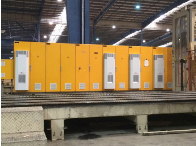
The electrical enclosures for the packaging line after being refitted with DTI cooling units.
