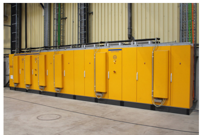
New switchgear cabinet for a short-cycle press for flooring manufacture, equipped with air/water heat exchangers from Pfannenber.
