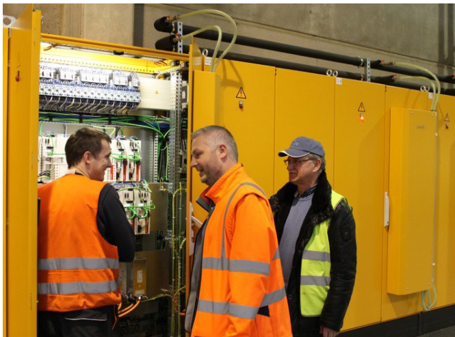
Discussion about a new electrical system: Frank Schmidt (centre) talking to his colleagues Rico Koßmann (left) and Werner Hille (right).
