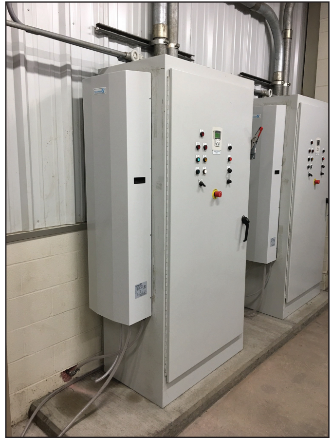
Pfannenber air-to-water heat exchange on a lift pump control panel at a wastewater treatment facility.
