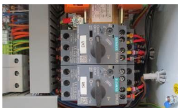
Picture 12– pump breaker On
