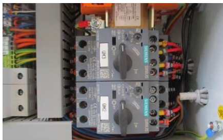
Picture 8 - Circuit Breakers
