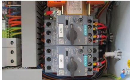
Picture 8 - Circuit Breakers
