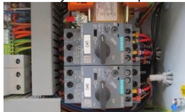
Picture 12– pump breaker On
